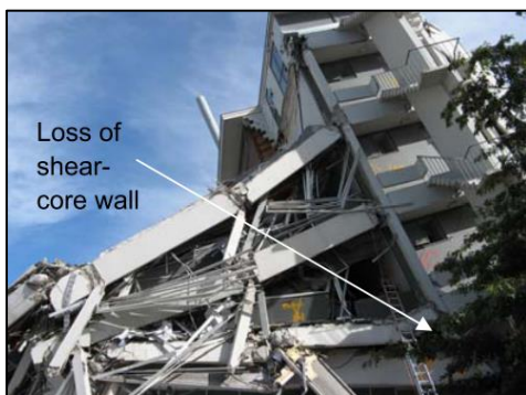
(k) Collapse likely initiated by axial failure of core wall [45]; PGC Building (1966)
