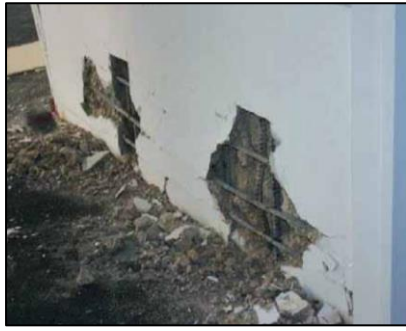
(e) Longitudinal reinforcement buckling; Canterbury Centre/Westpac Tower (1981) (source: Spencer Holmes)
