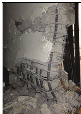
(i) Out-of-plane movement and instability of wall; 123 Victoria St (1980-1989)
