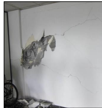
(d) Concrete spalling at web to boundary element interface; BNZ Tower (1967) [43]
