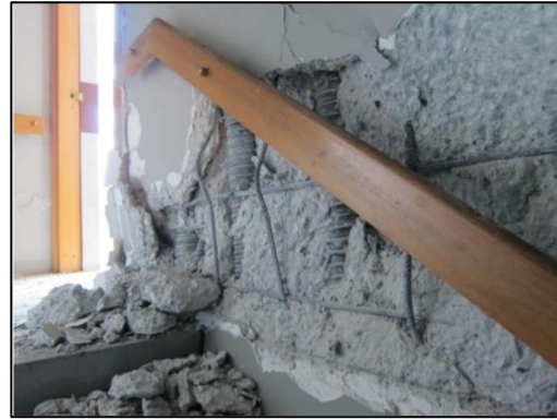
(n) Buckling of longitudinal reinforcement and spalling revealing grouted duct splice connection in precast wall; Crowne Plaza Hotel (1980-1989) [44]
