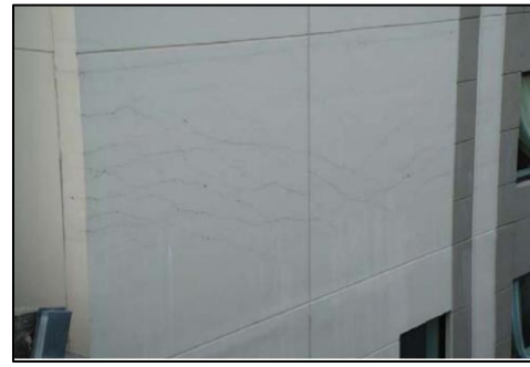
(b) Well-distributed cracking; Novotel building (2008-2009) [42]
