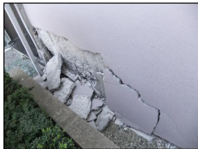
(g) End region core crushing; Terrace on the Park (2000-2010)
