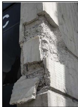
(c) Spalling of cover concrete; Crowne Plaza Hotel (1980-1989)
