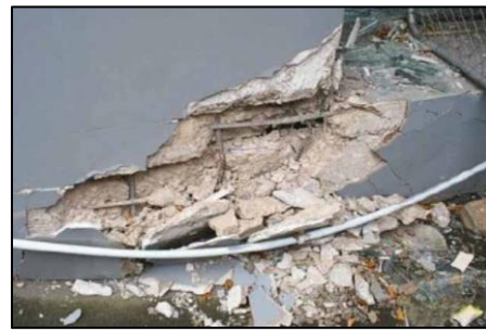
(h) End region core crushing and reinforcement buckling; AMI Building (1970-1979) [44]
