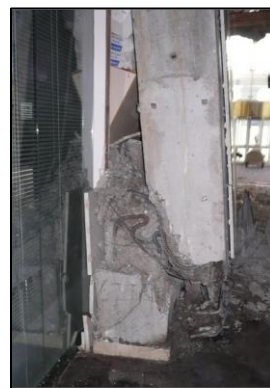
(j) Shear-axial failure of wall; Hotel Grand Chancellor (1985-1988)
