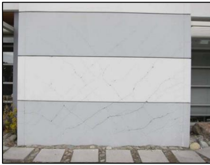
(a) Well-distributed cracking; NZ Statistics House (1999-2000)
