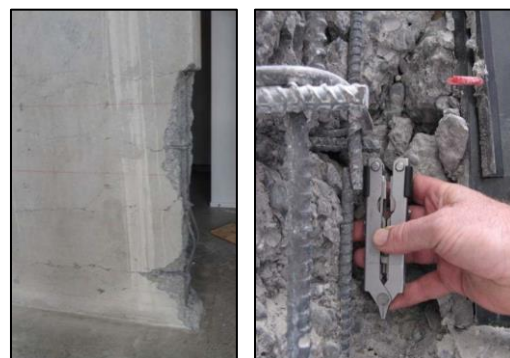
(l) Localized longitudinal reinforcement buckling and tensile fracture; Gallery Apartments, (2005-2007)
