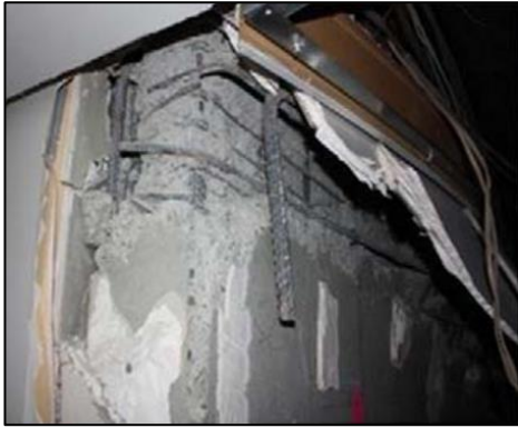
(m) Loss of horizontal reinforcement anchorage after cover spalling; Terrace on the Park (2000-2010)
