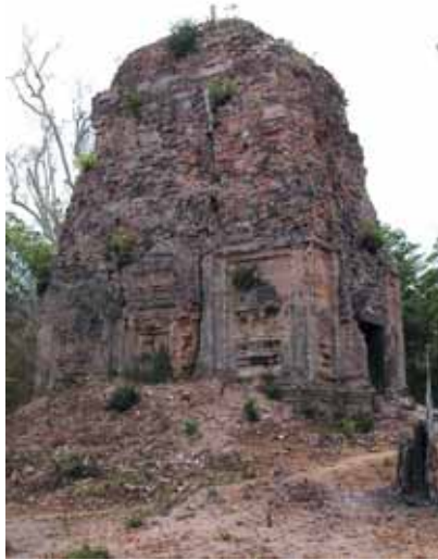
Figure 7. Vertical crack at the middle of wall (N21 shrine in Prasat Sandan, M.10).
