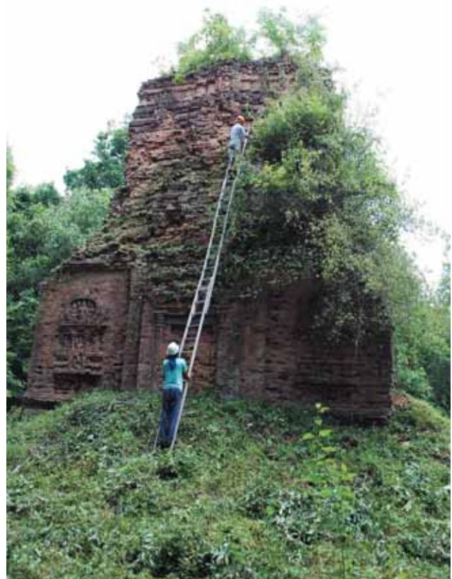
Figure 3. Removing vegetation on the brick structure as the periodical maintenance activities at N15 shrine.
