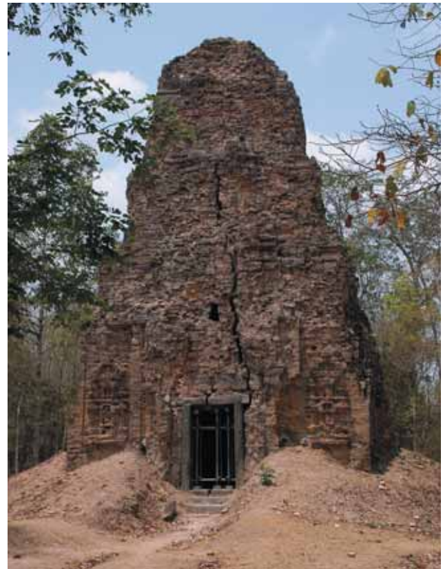
Figure 6. Collapse around and above door opening (N11 shrine in Prasat Sambor, M.20).
