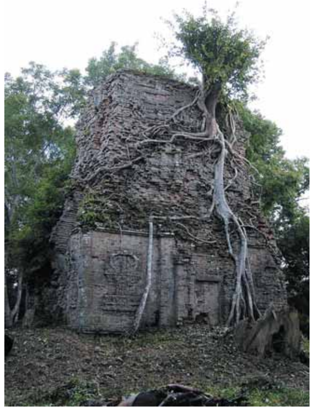
Figure 11. Loose and fragmentation of brickwork of roof part (W shrine in Prasat Kouktroung, M.41).
