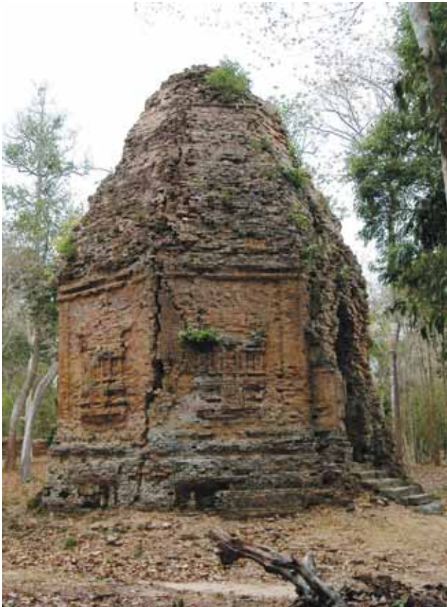
Figure 8. Vertical crack at the corner of wall (S7 shrine in Prasat Yeai Poeun, M.24).
