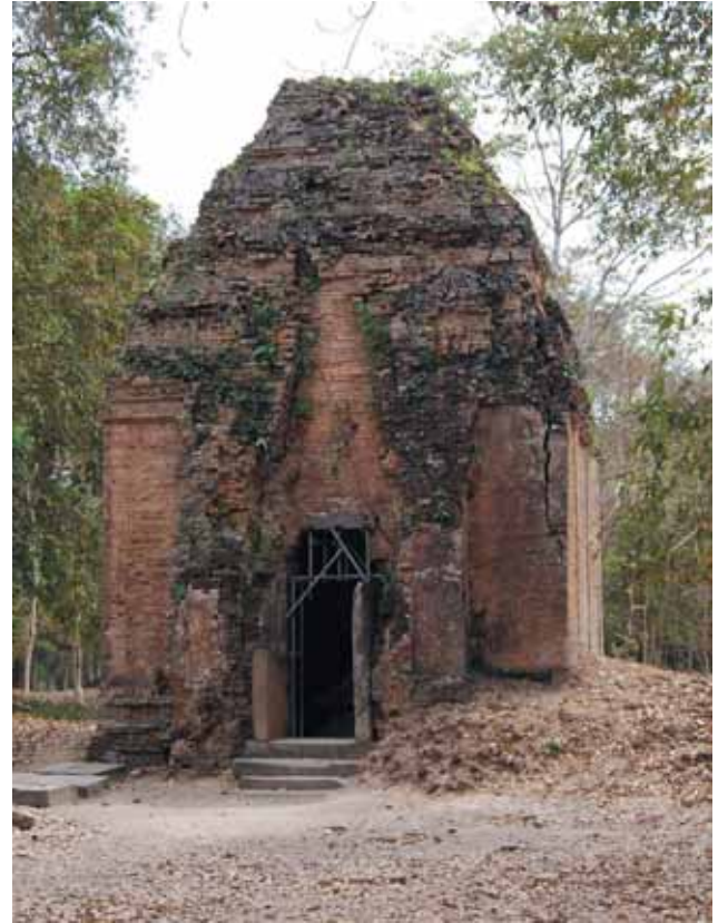
Figure 9. Crack at the corner of wall (N10 shrine in Prasat Sambor, M.20).
