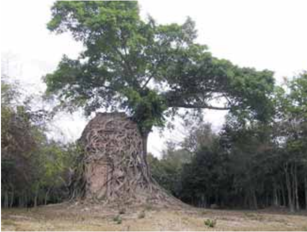
Figure 2. One of the brick structures with growth of tree (N18 shrine, Prasat Chrey, M.17).
