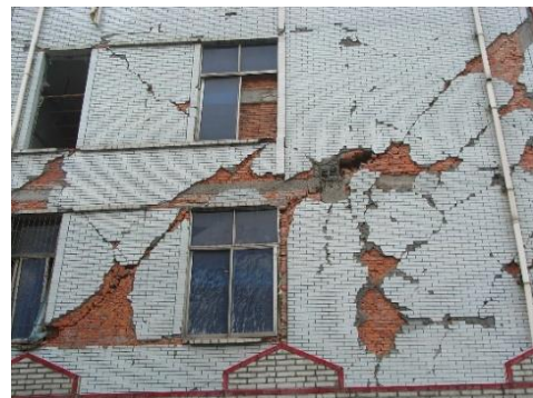
Figure 1: Damage of RC building with masonry infill walls in China 2008 Wenchuan Earthquake.
