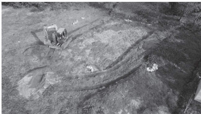
Figure 12: Overhead view of Suwahara site as excavator finishes returning the sand and soil to the excavated pit. (19 November 2020)
